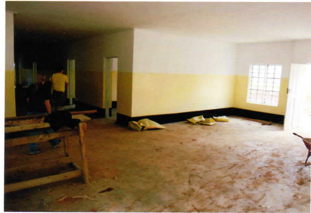
Above - Finishing up the interior of the new AIDS CTC (Care & Treatment Center) building. Jenny Peck—Feb 2010
